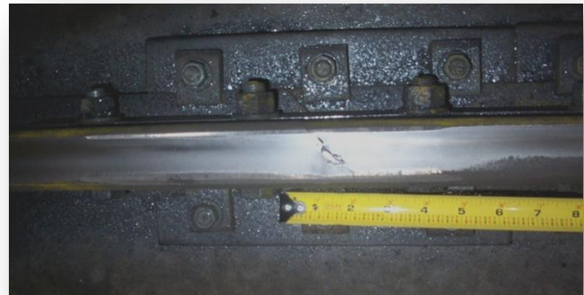
Flat and Damaged AS/RS Floor Rail Splice Joint
